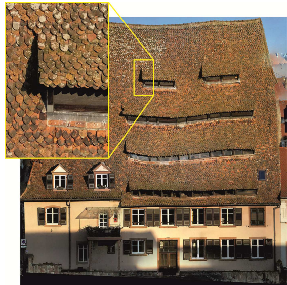
Figure 7: Example of a produced Orthophoto captured by UAV of the "Maison du Sel" before the reconstruction of the roof with a resolution of a 5 mm GSD.
