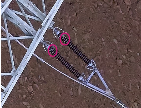
Figure 8: Image with detected insulator Issues on a X-pole along an observed powerline
